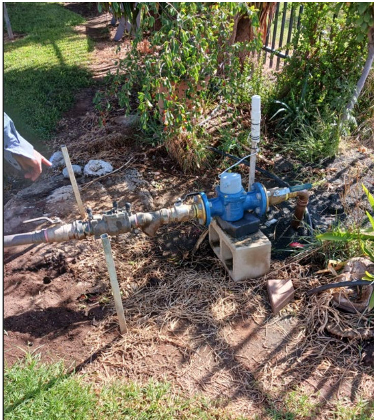
Figure 2: New Smart Meter installed at a property in Narromine
